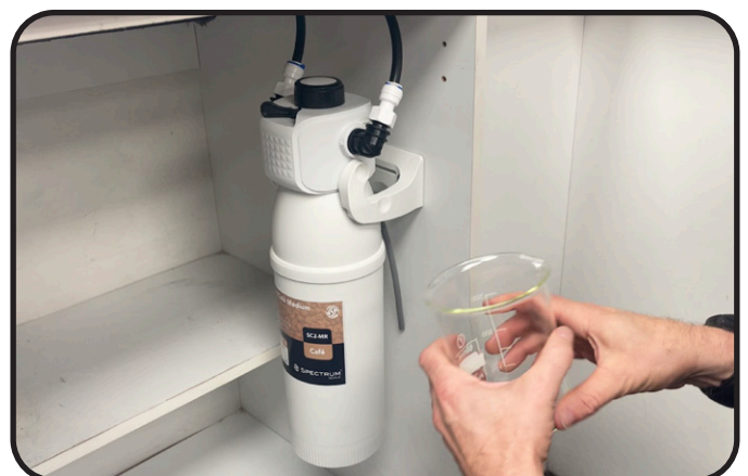
(Complete unit fitted in cupboard.)
